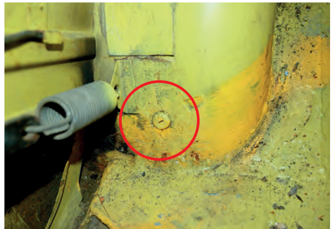
The later positioning of the outside mounting point, just inside and below the tonneau spring bracket. The insert is normally black but has been oversprayed yellow in this car.
